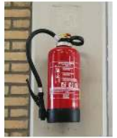
This is a fire extinguisher
